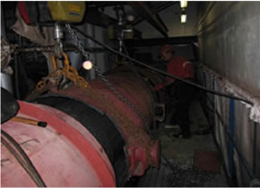
Existing Tubular exchanger LEL1 in situ
